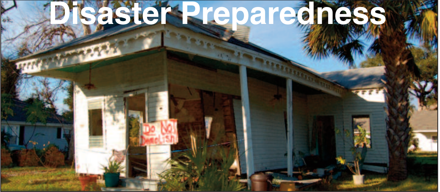
A historic Mississippi Gulf Coast beach cottage damaged by Hurricane Katrina. NPS photo.
