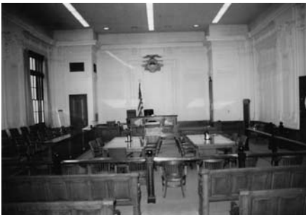
FIGURES 5-6 GSA Building Preservation Plans identify spaces of architectural importance and character-defining features to be preserved and restored, such as this hidden ornamental ceiling restored as part of the building systems upgrade.
