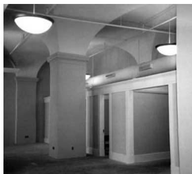
FIGURE 10 Thoughtfully exposed ductwork allows vaulted ceilings to remain exposed to view.
