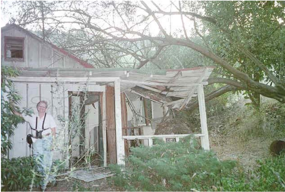
Plate 2. East elevation of cabin before porch was removed for repair. Facing west. 2002. Courtesy Linda Dye
