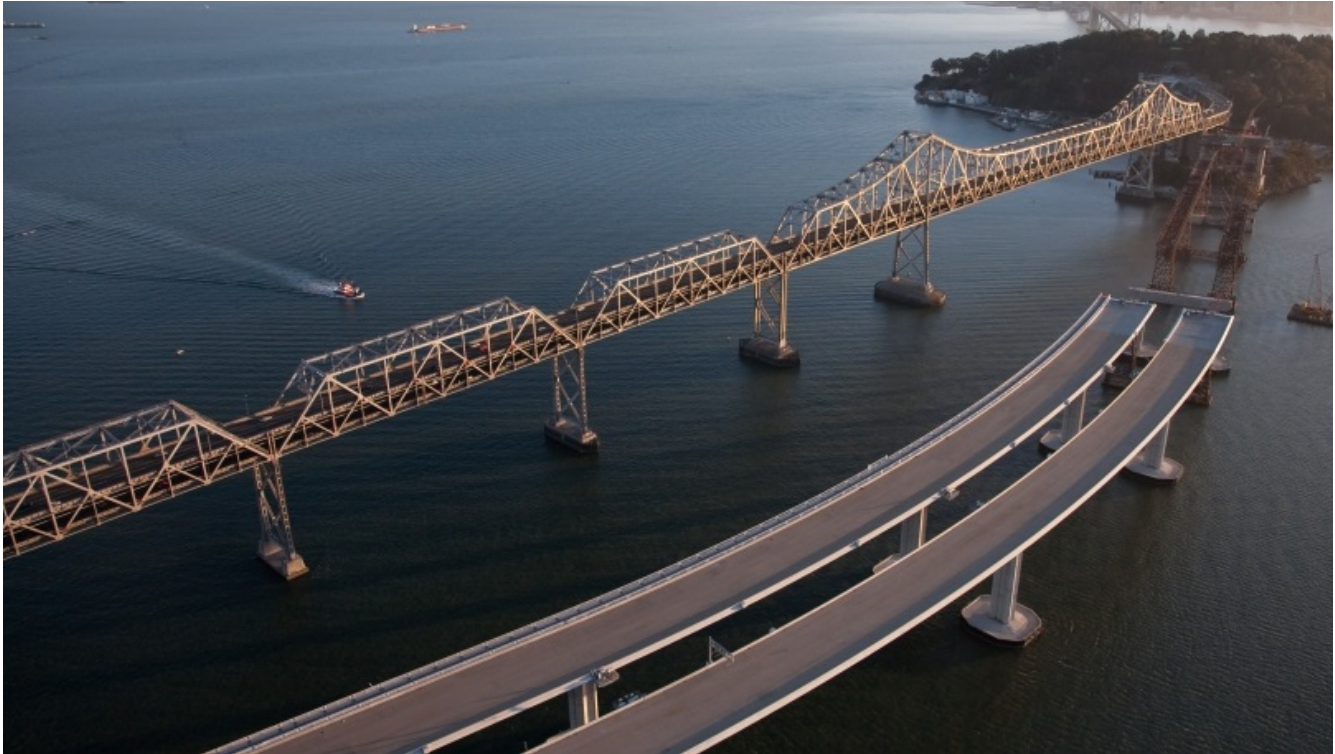
Figure 7: Skyway under construction to the north of the original bridge structure. Undated Caltrans photo, baybridgeinfo.org, accessed 4/27/2020.
