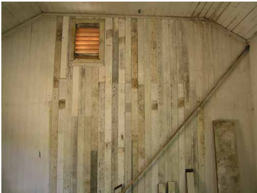
Interior View of Cambria Chinese Temple (South Wall) Following Wall Cladding Repairs and Prior to Paint Restoration Photo Taken Ca 2007
