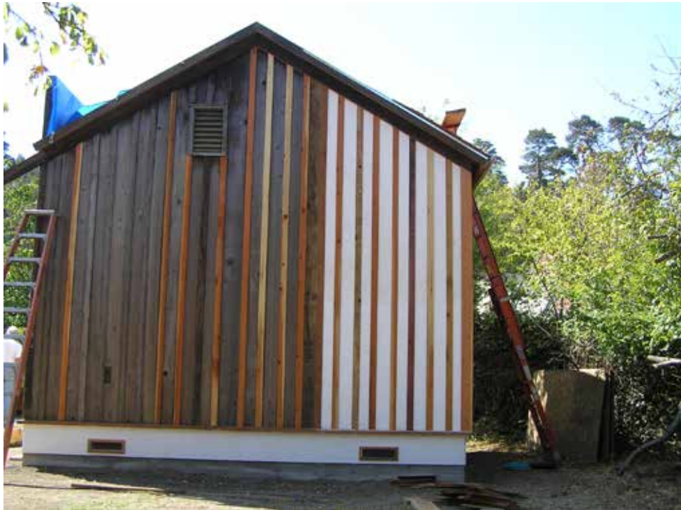
North Elevation of Cambria Chinese Temple Following Siding Repair Photo Taken Ca 2007
